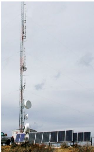
Thompson High School tower on a 7,000-foot mountain and powered by solar
